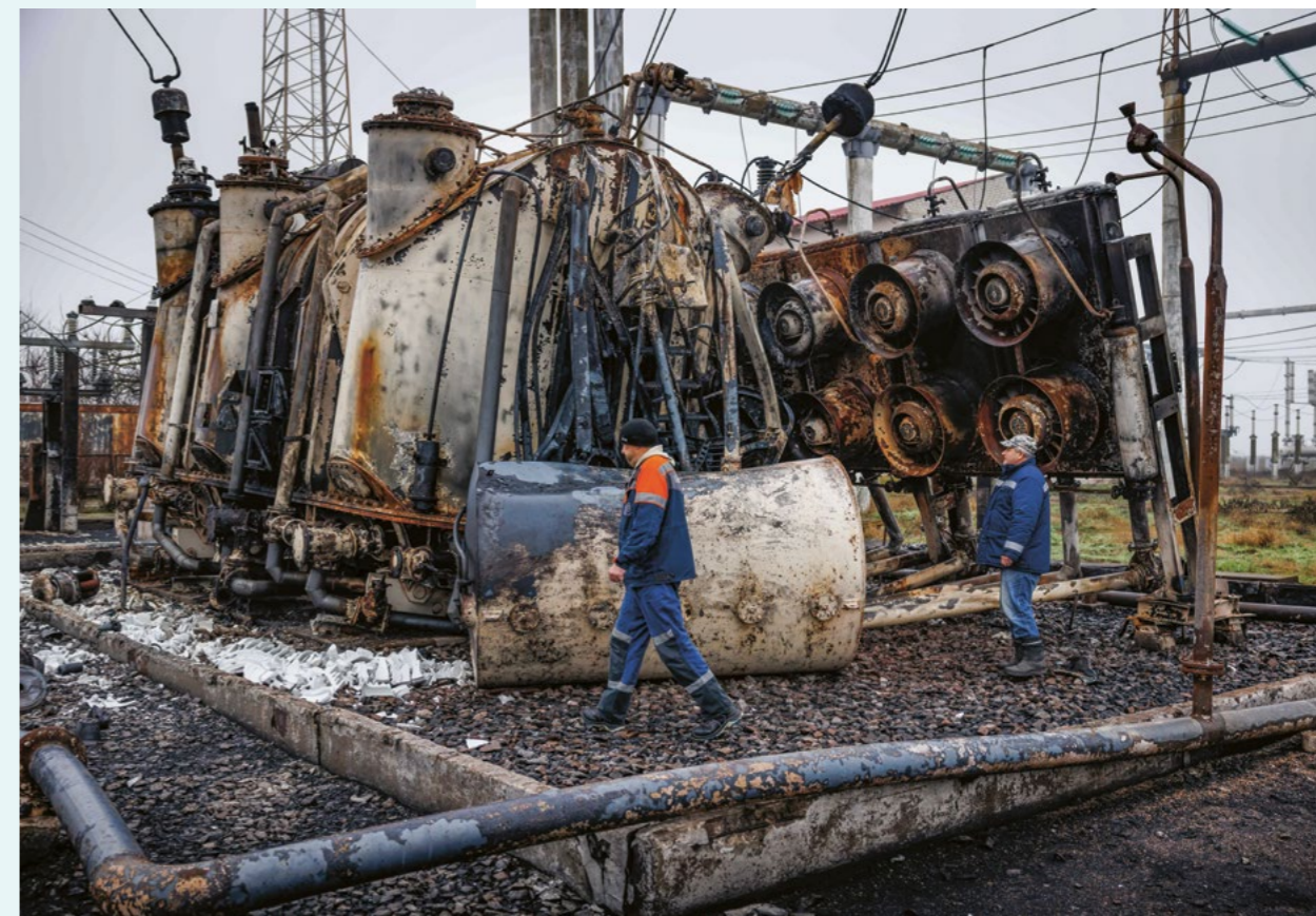
A transformer in Kherson that has been destroyed by Russian troops. Russia's attacks are aimed at Ukraine's critical infrastructure.
