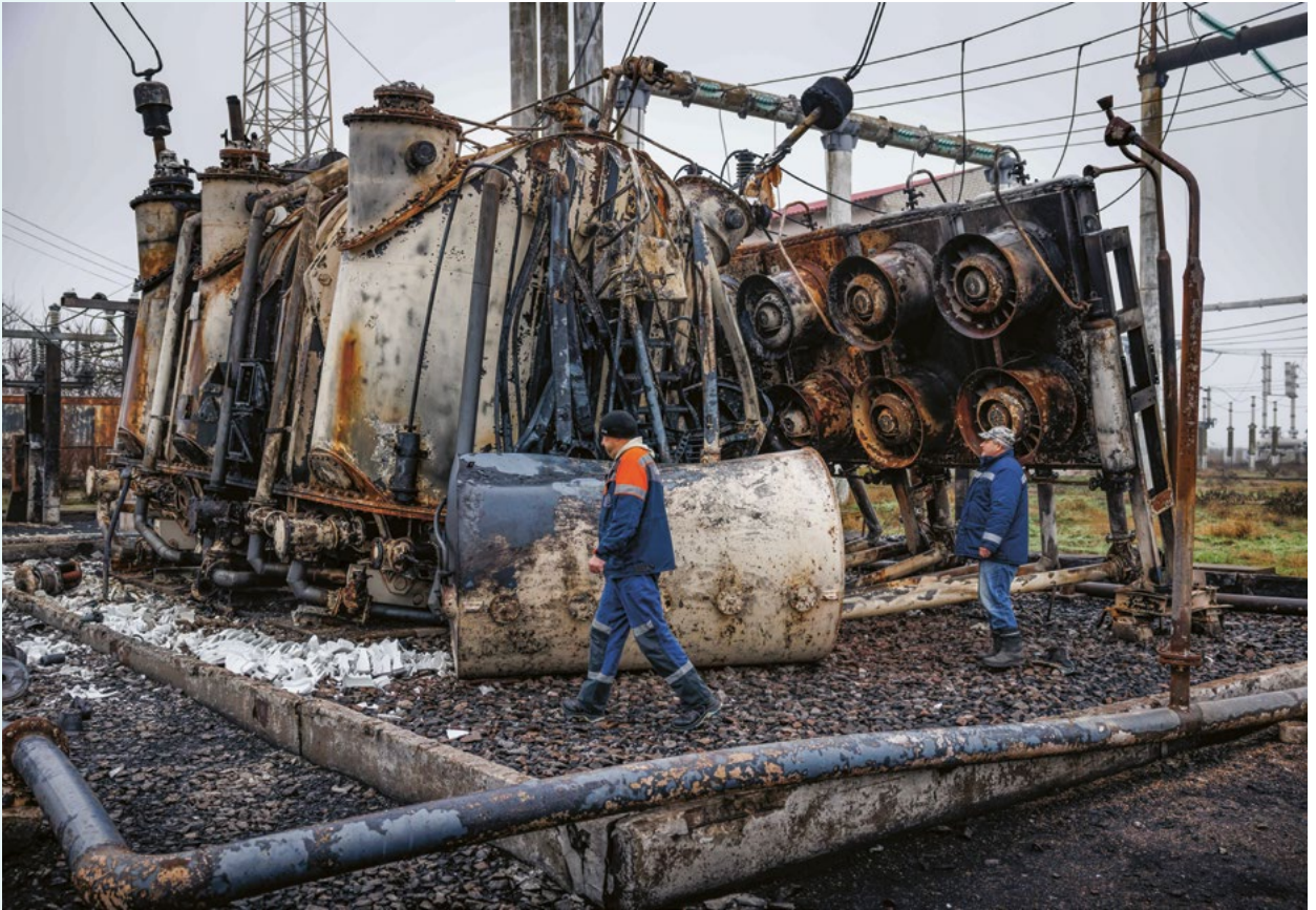
A transformer in Kherson that has been destroyed by Russian troops. Russia's attacks are aimed at Ukraine's critical infrastructure.
