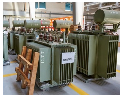
Partner donations: transformers for Ukrainian substations
